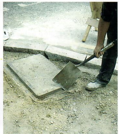
Inspection covers often need to be adjusted
