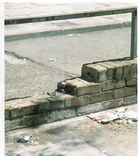
Landscape walls need to be maintained
