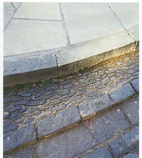
One of the variations of sett drainage channel
