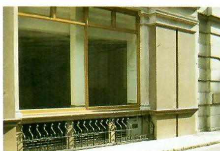
Wall mounted lighting & switch box
