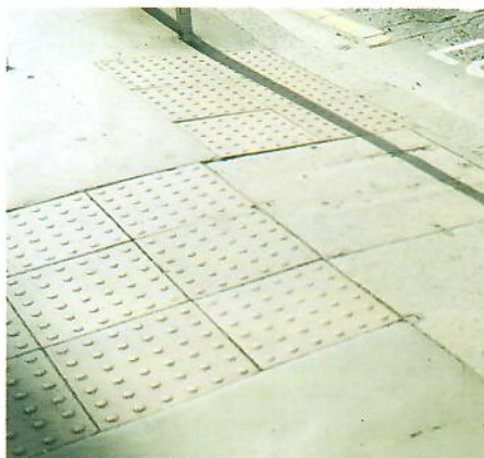
Tactile surface distorted by inspection covers
