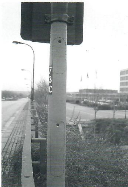
Two access panels in column, Milton Keynes
