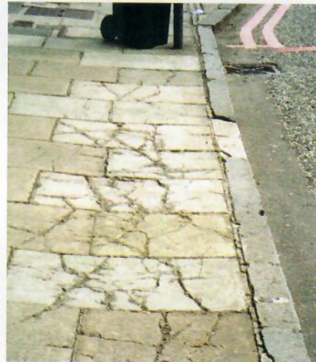
Cracking up under the strain: Damage to footways caused by heavy goods vehicles is a common sight in urban streets throughout the UK. ( Below ): Students from the Institute of Highways Incorporated Engineers, in a series of experiments, tested various paving stones for strength. Steel-reinforced slabs proved to be the most resilient
