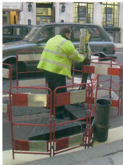
Underground telephone cable cabinet
