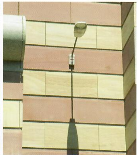
Wall mounted lighting on modern building
