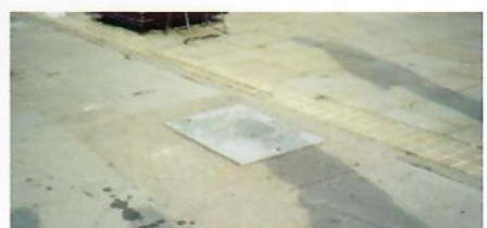
Electricity supply cabinet for street market
